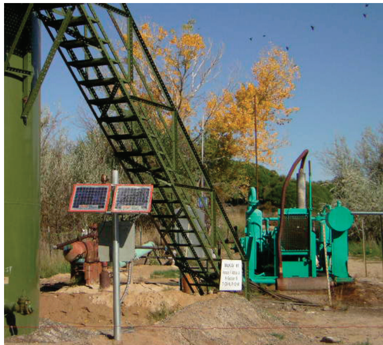
Wellkeeper monitoring equipment on McKay gas well
